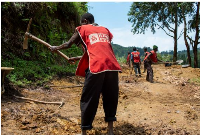
Cash for Work to maintain roads in DRC – important source of income for conflict-affected people, and key to communities to access markets, health care, schools, etc.
